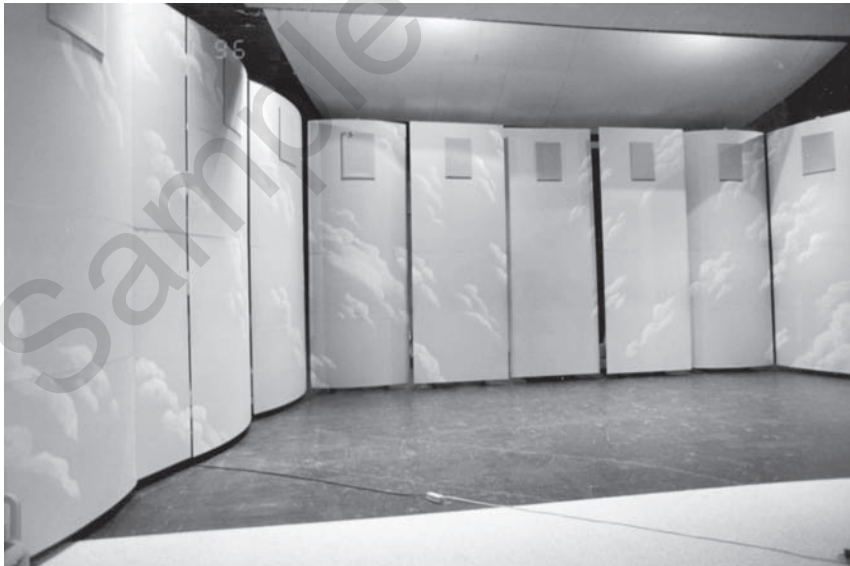
Figure 6.10 Using an electronic reverberation enhancement system one can achieve high flexibility in room acoustic conditions. The photo shows an active system for control of acoustics on a stage using loudspeakers integrated into a stage shell to achieve a proper blend of early reflections and local reverberation. Installation in Motala Community Center, Sweden. (Photo by Mendel Kleiner.)
