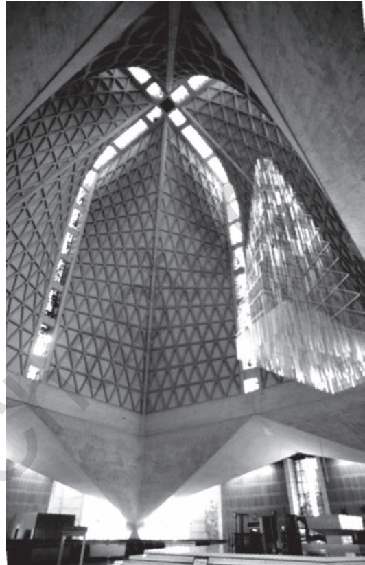
Figure 6.6 When the sound absorption of the walls is high, a room having high concave ceilings is susceptible to echoes. The ceiling in this church has been made extremely irregular to scatter sound and avoid echo. (Photo by Mendel Kleiner.)
